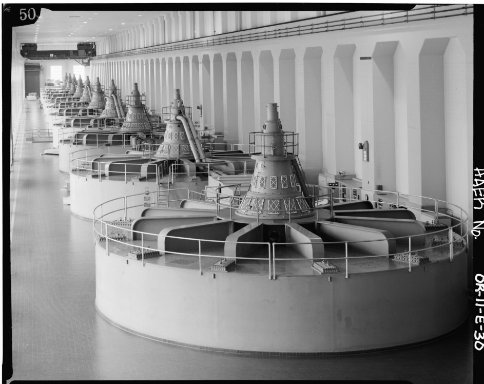
Fig. 6: Interior View Of Powerhouse One. National Parks Service.
