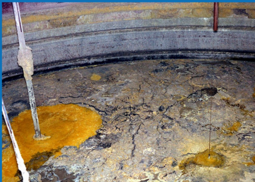
Image of the inside of an underground tank at Hanford Image courtesy Oregon Department of Energy
