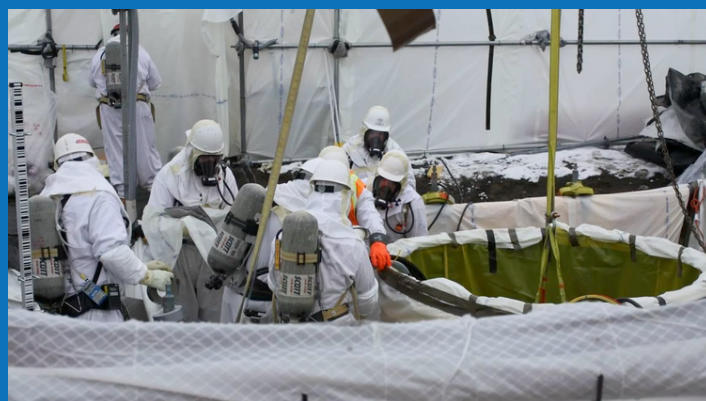
Image of Workers removing radioactive waste at C Farm Tanks Image courtesy Washington River Protection Solutions
